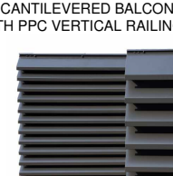
12. POWDERCOATED MILD STEEL LOUVERED GRILLES FOR VENTILATION
